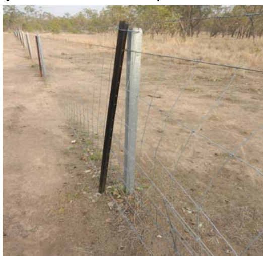
Photo 11: Used Maxi posts in floodways to allow the fence to move with water flow
