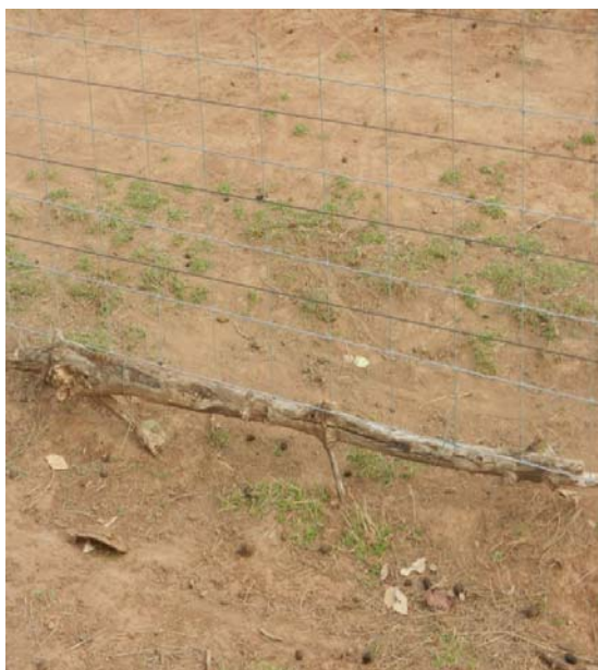
Photo 10: Logs have been tied in any spots where old roo holes existed
