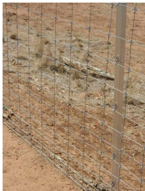
Photo 8: Fence 2 – Clipex™ post were used which made it easy to attach the wires
