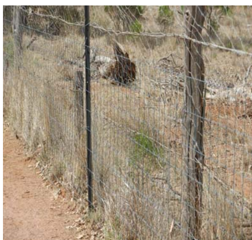
Photo 4: Fence 1 - The new fence was run alongside and tied to the existing old wild dog netting fence
