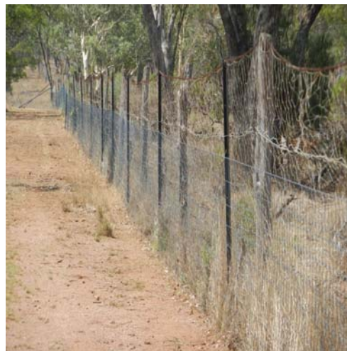
Photo 3: Fence 1 - The existing wild dog netting was tied to the new steel pickets
